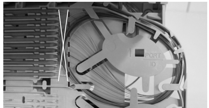
9.5.9. Wrong installation of loops around the island. Loops are passing the line and are too close to the splice holder.
