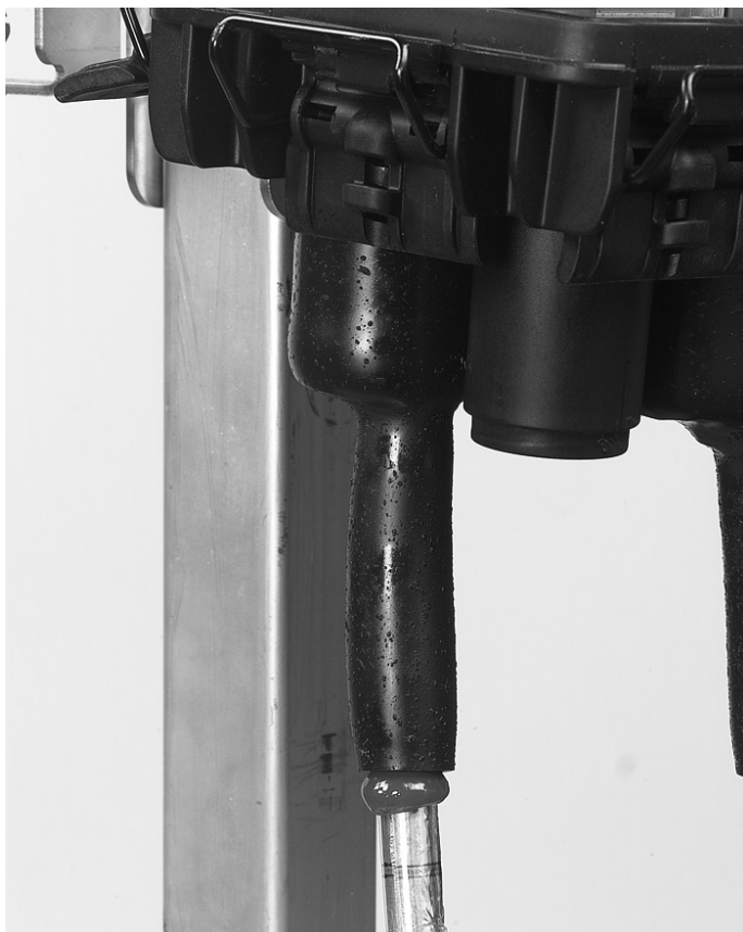
8.2.2.4. Drop cable sleeve installed.
