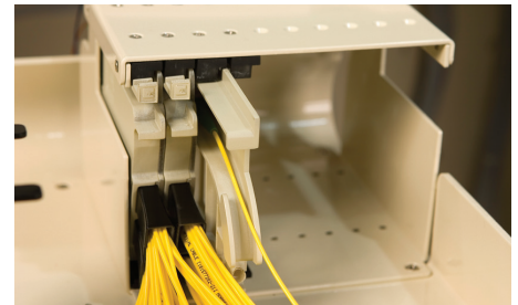
Feeder Pass-Thru Feature
